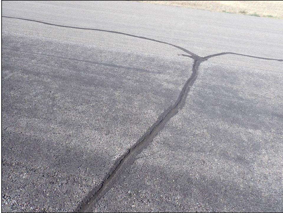
RW06-01-06: L&T Cracking
