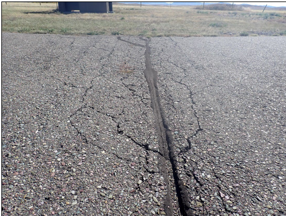
AP-01-03: Alligator Cracking
