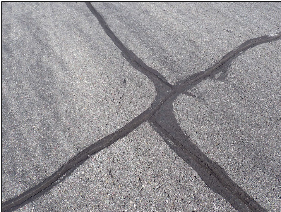
RW06-01-53: L&T Cracking
