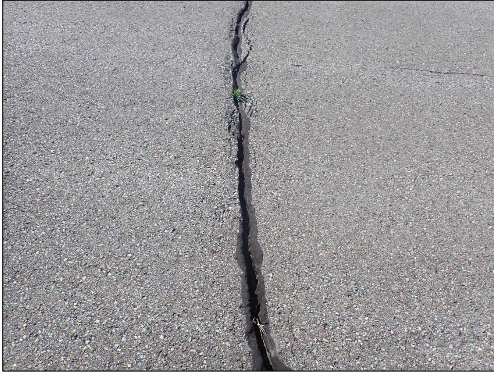
AP-01-02: L&T Cracking
