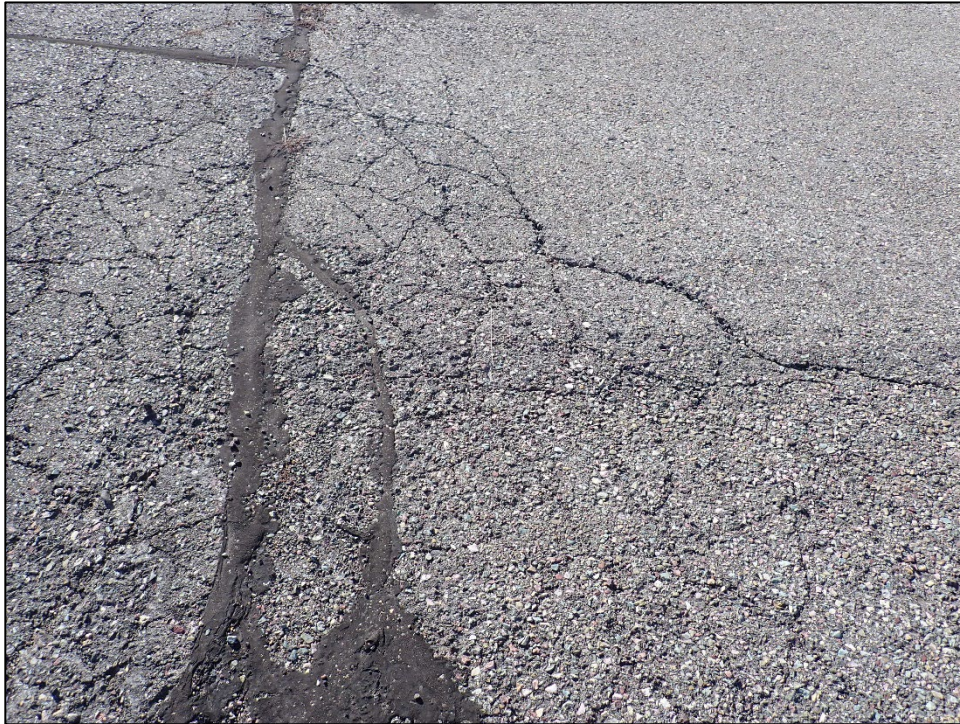
TW-01-01: Alligator Cracking
