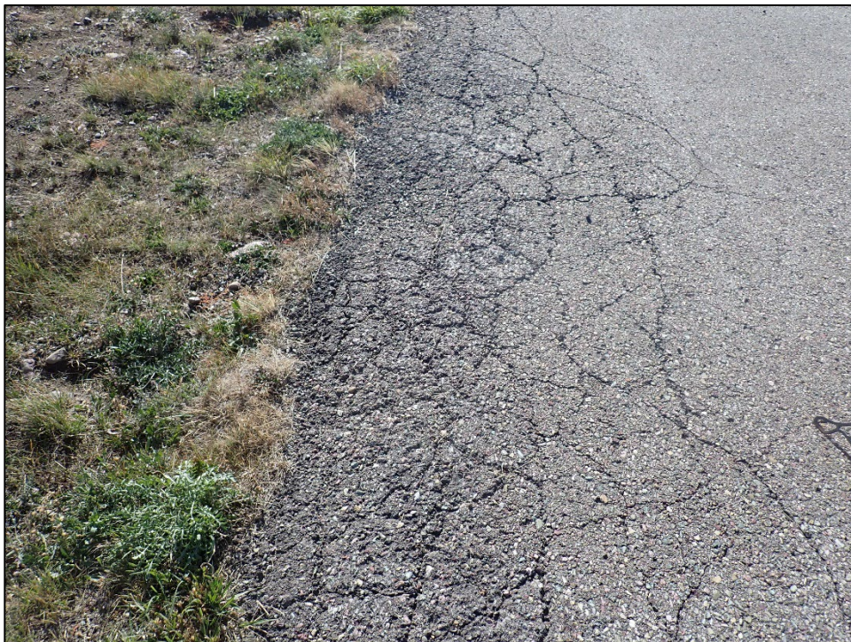
TW-02-03: Alligator Cracking
